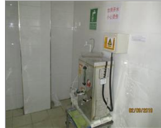
Photo of the sanitary facilities Drinking water.JPG
