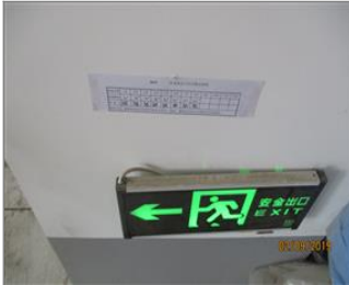
Photo of fire safety equipment Evacuation sign.JPG
