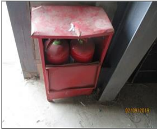
Photo of fire safety equipment Fire extinguishers.JPG
