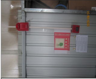
Photo of fire safety equipment Fire alarm.JPG
