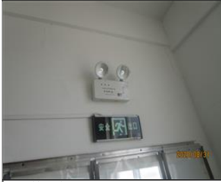
Photo of fire safety equipment Emergency light and sign.JPG
